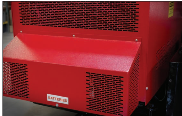
BATTERIES STORED HERE
